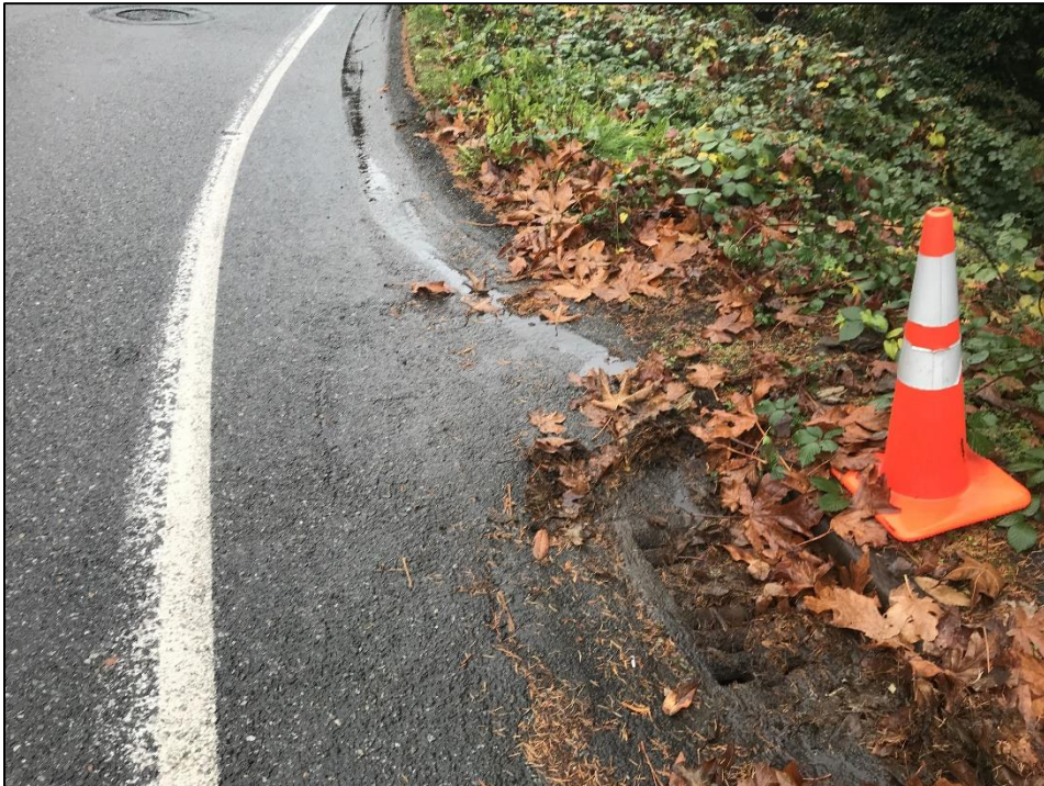
Photo 3. Visible stormwater input to stormwater grate with connection to black PVC stormwater main.
